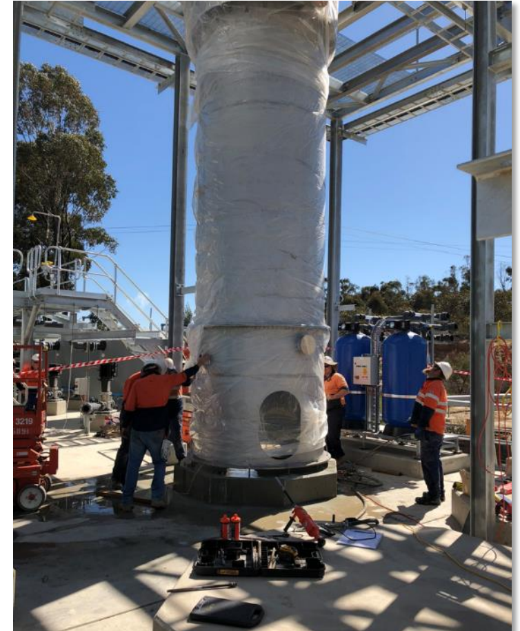
Ion-exchange columns installed at Fosterville Gold Mine
